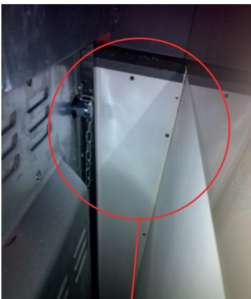
Left side of the oven: Chain not attached.
